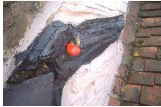
Probing with a screwdriver locating severe decay behind impervious paint
